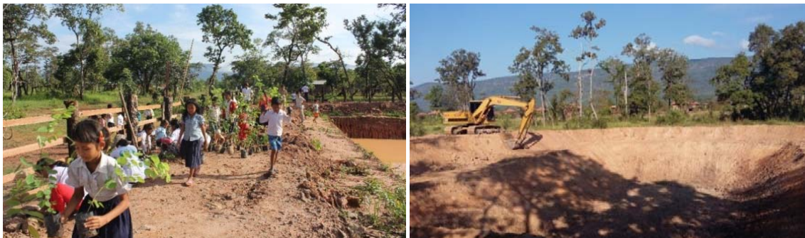
The digging of a pond to reserve water for school and community consumption during the dry season.
